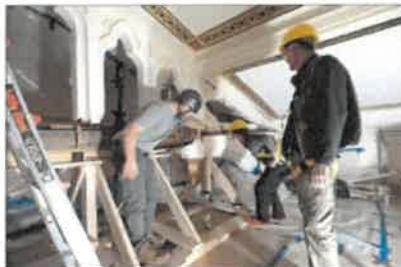
Ken M. Saul Jr. of Restoration Artisans in Kutztown, left, points out details that need repair to Alex O'Gorman and John P. Wood of the Pennsylvania Historical and Museum Commission at Christ Episcopal Church. BILL UHRICH/READING EAGLE
